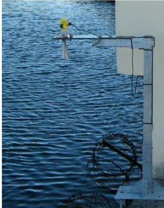
Figure 22: Example of a radar sensor installed above a river
