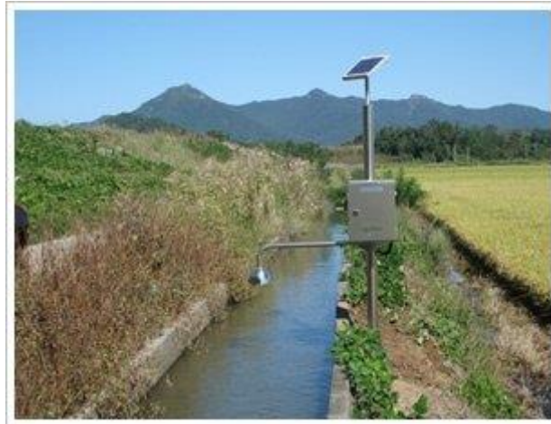
Figure 21: Example of an ultrasonic sensor installed above a canal
